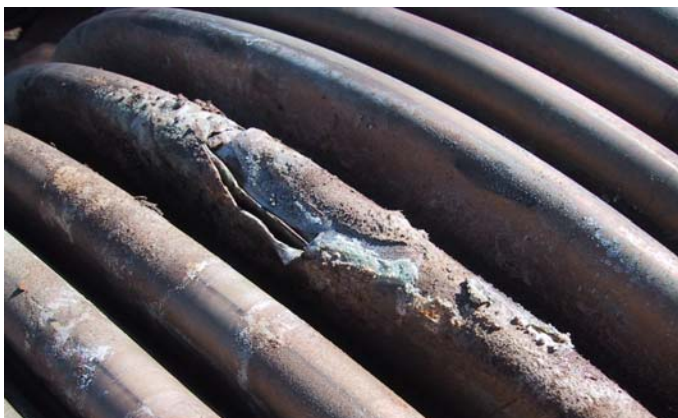
A distorted cover opened up this bellows like a can of sardines
